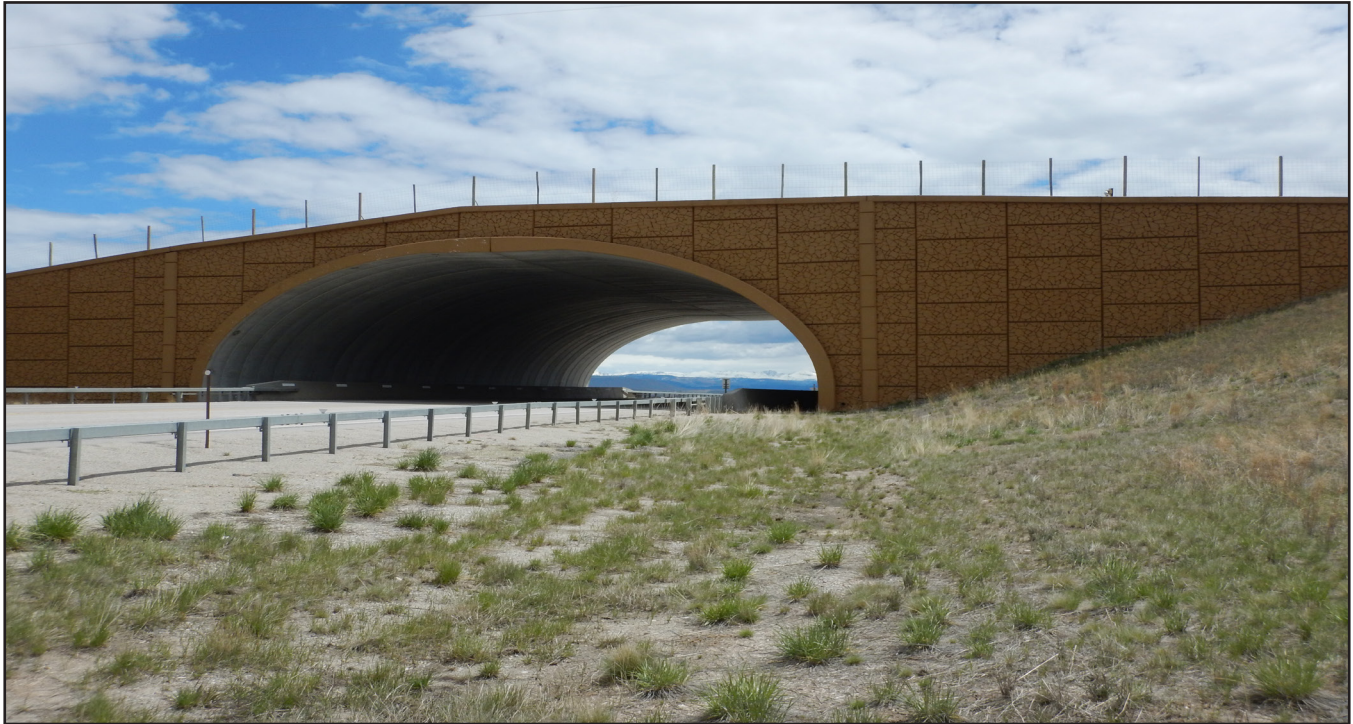
A wildlife crossing structure at Trapper's Point in Wyoming over U.S. Highway 191.
